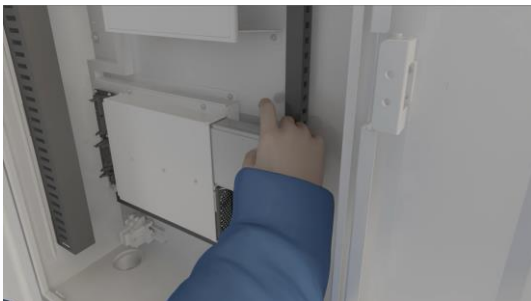
Main control module hot swap maintenance
